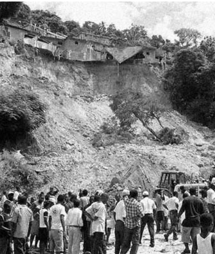
Rebuilding work begins after a landslide in Port-au-Prince, Haiti. Photo: Michel Matera/UNDP
